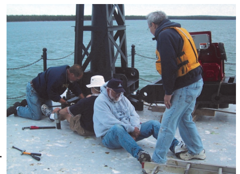
Re-installing the second crane: Ed Clark, Dave Bardsley, Meade Gable, and Don Gries
